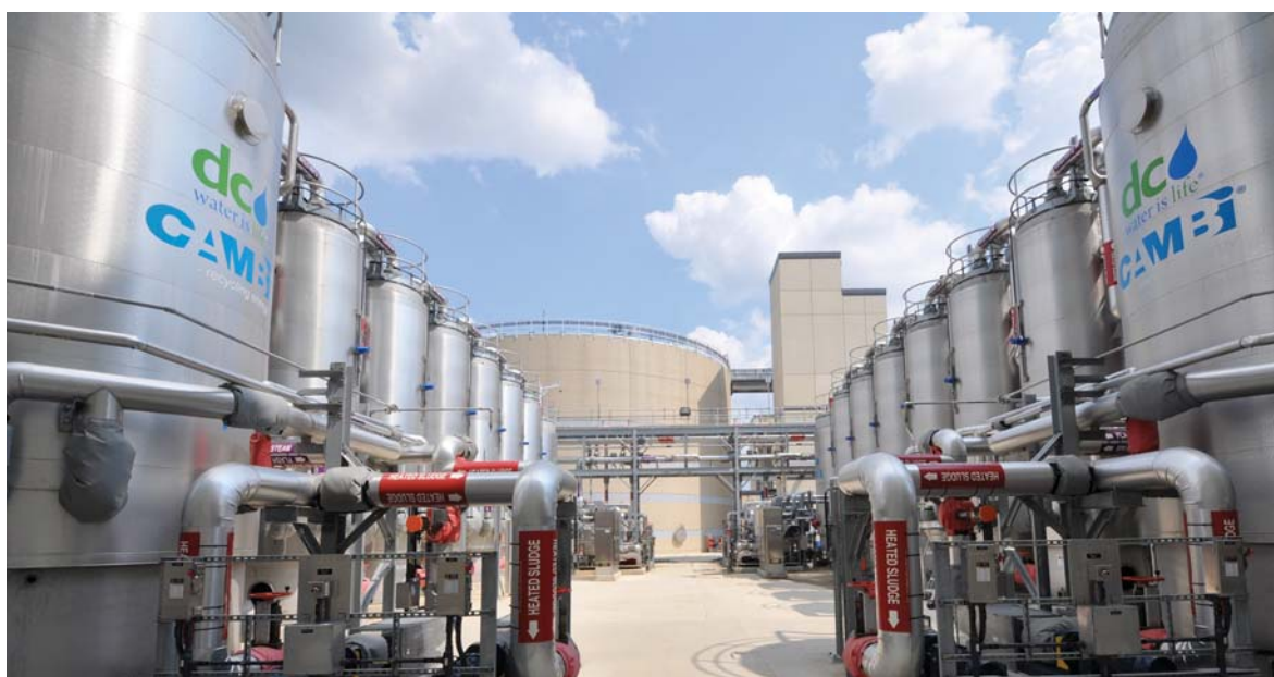
Part of the combined heat and power bioenergy plant at the Blue Plains Advanced Wastewater Treatment Plant, District of Columbia, USA. Photo: DC Water
