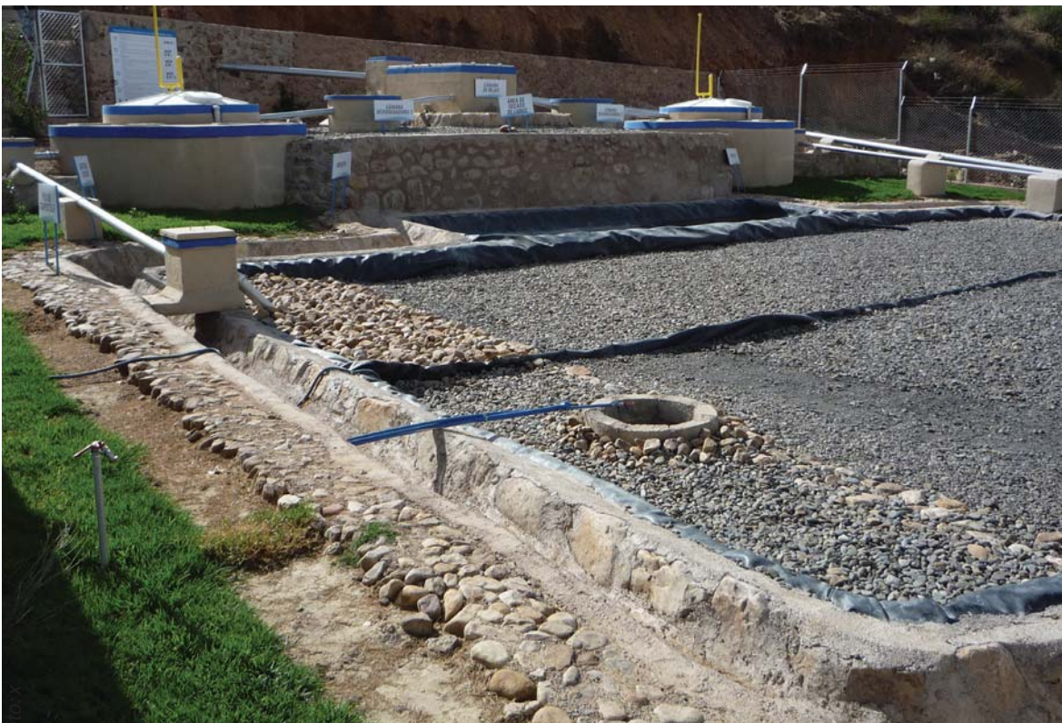
Decentralized wastewater treatment plant with constructed wetland, Cochabamba, Bolivia. Photo: Kim Andersson
