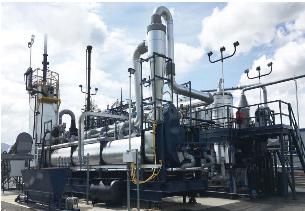
A combined heat and power plant that recovers energy (heat and electricity), potable water and ash from faecal sludge and other combustible waste. Photo: Flickr / SuSanA Secretariat / Janicki Bioenergy
