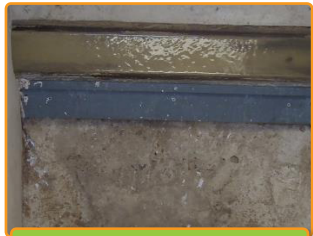
Stormwater overflow installed at head of Newlands Mashu DEWATS plant.
