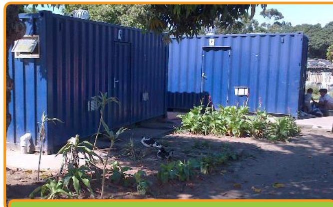
Photograph of community ablution blocks connected to ABRs in the Frasers settlement. Photo by Bjoern Pietruschka (2014).
