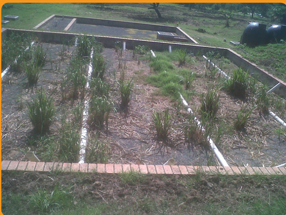
The wetland modules of the Newlands Mashu DEWATS plant. The vertical flow constructed wetland (middle) is fed through a siphon filter. The horizontal flow constructed wetland is shown on the top (wetland was not planted when photograph was taken in February 2012). Both wetlands were planted with vetiver grass.
