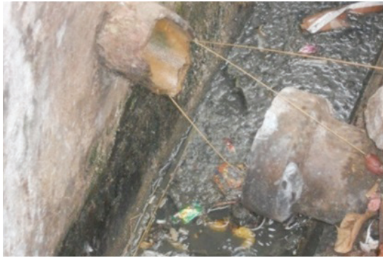
Toilet directly connected to open drain
