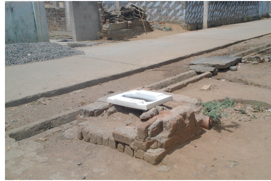
Dysfunctional pit latrine
